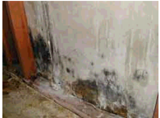
Mold growth behind laundry wall.
